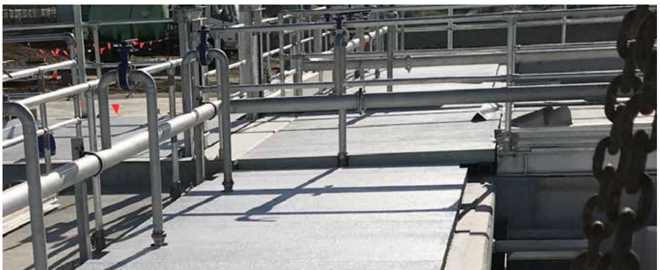
SureLine® & various hatch types. Queensland, Australia.
